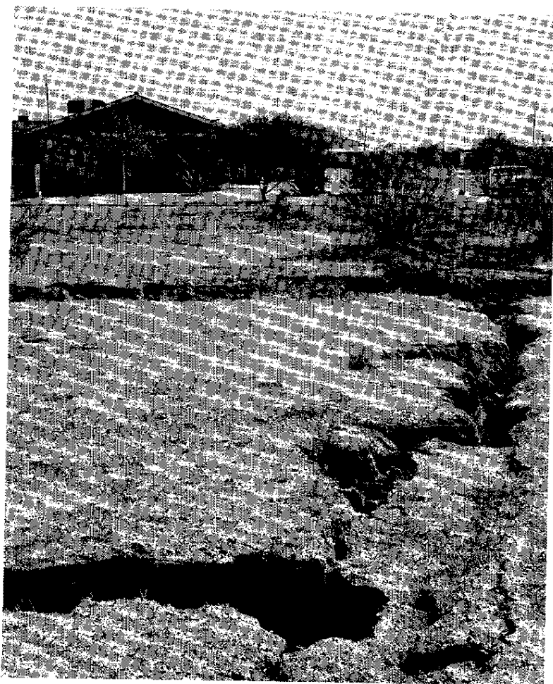
Homes endangered by a mile-long earth fissure. Perpendicular gullies are occurring by piping and erosion (E. E. Hertzog, Bureau of Reclamation).
